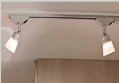
Halogen uplighters and 12 V reading spot lights Have light where you need it. The angle of the spotlights can be adjusted and freely moved along the track.
